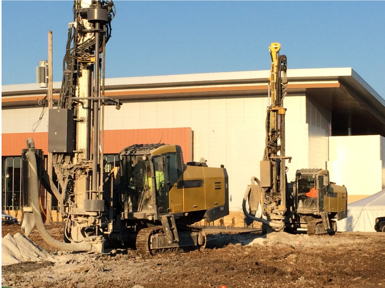
Figure 4-5. Two Air-Percussion OHD Drill Rigs. Note Pile of Rock Fines (Drill Cuttings) in Front of the Rigs Removed from the Hole.
