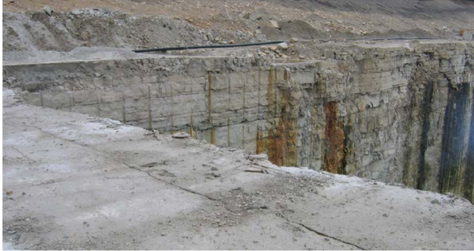
Figure 3-7. Tension Crack in Rock Mass after Presplit Blasting.
