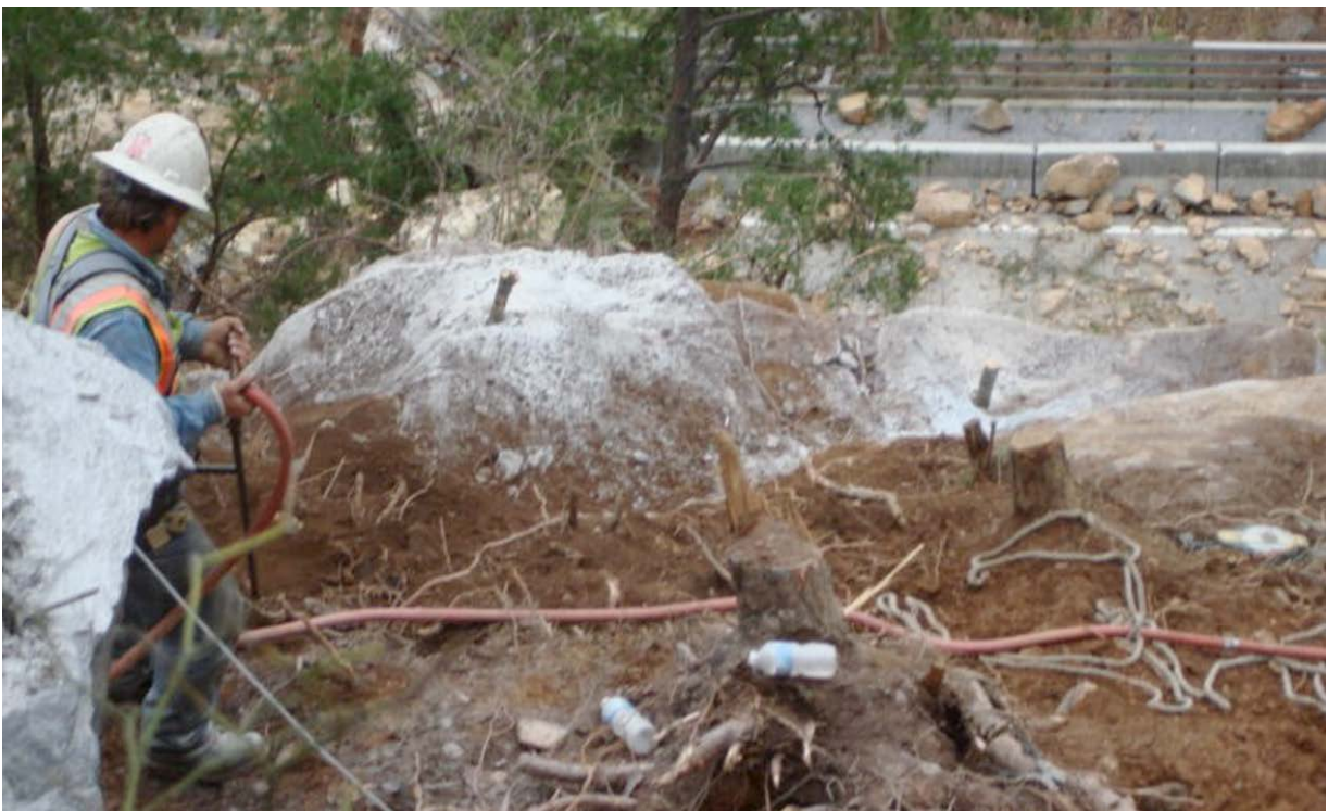
Figure 4-3. Photograph of Air Rock Drill Used for Blasting of Boulders on a Rock Slope.
