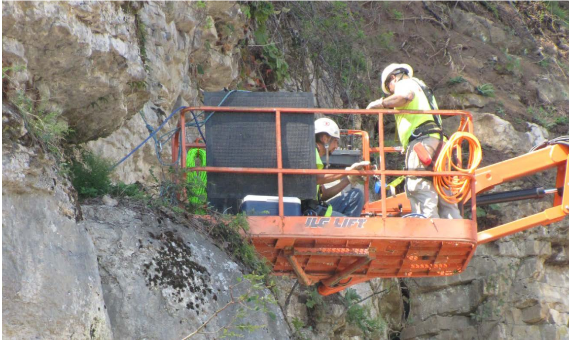
Figure 6-21. Airbag with Scalars in a Man Lift before Being Placed behind a Large Unstable Column of Rock to Be Removed from a Slope.
