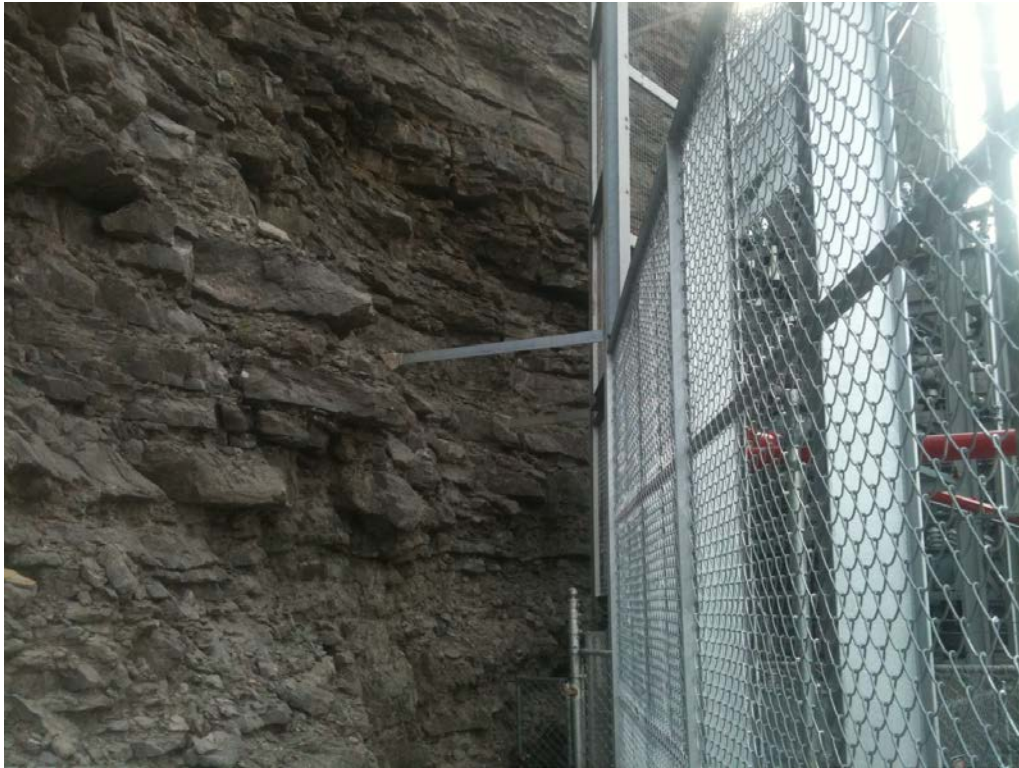
Figure 6-1. View of Rock Slope Next to Switchyard with a Problem Face. Note that the Fence Was Installed To Protect People and Switchyard Equipment from Rocks Falling from the Wall.
