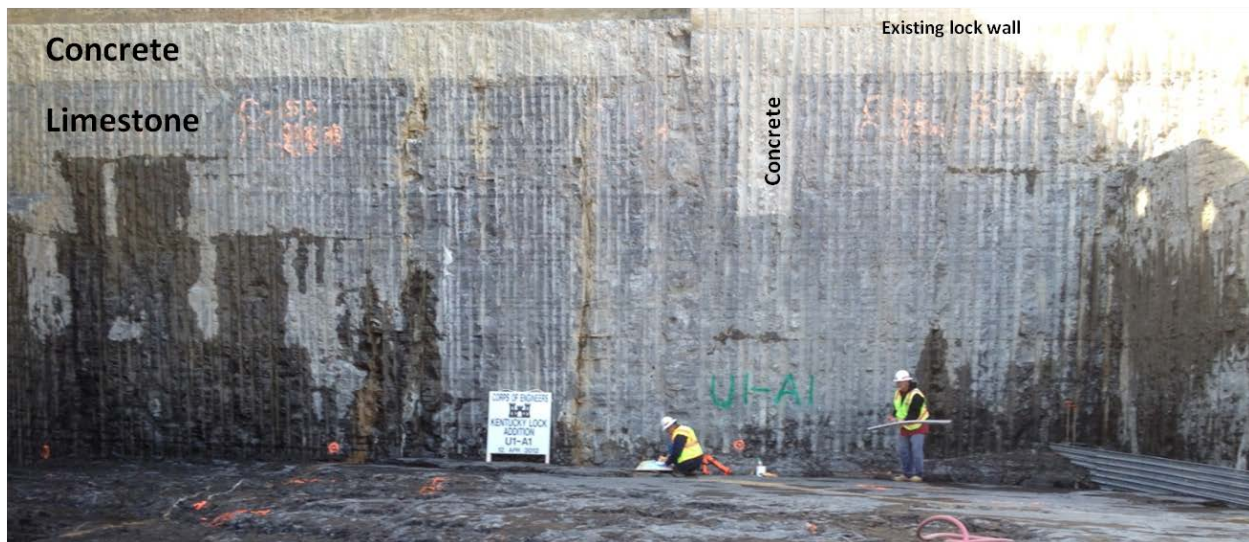
Figure 6-6. Line Drilling at Kentucky Lock Project Used for Construction of Excavation for New Lock Chamber Located Adjacent to and Immediately below the Existing Lock Wall.
