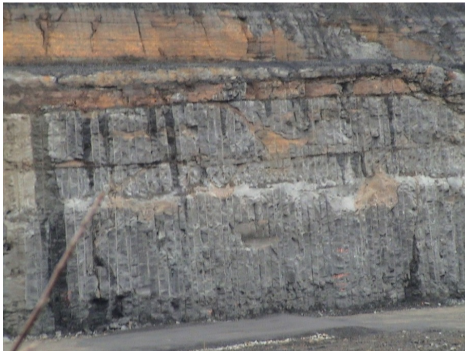
Figure 6-8. Over 1.5 Million Feet of Detonating Cord used on USACE Precision Presplit Project, Grundy, VA.
