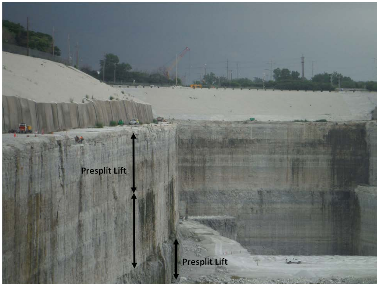
Figure 6-5. View of Highwall Excavation in Limestone Using Presplit Blasting with up to 125 ft Presplit Lifts.
