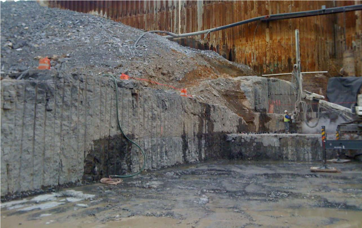
Figure 4-1. View of “Half Casts” on Rock Slope after Blasting at Kentucky Lock.
