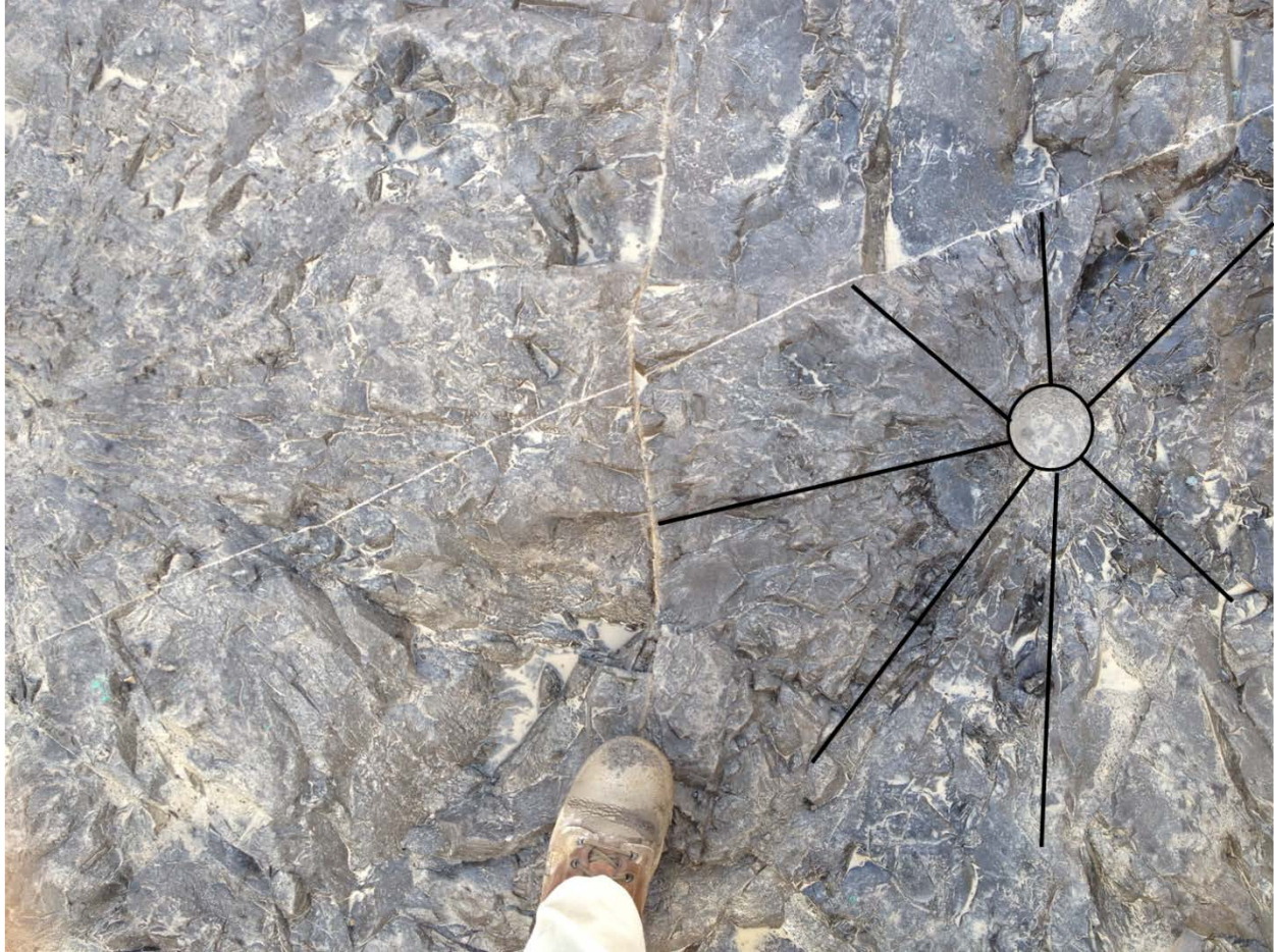
Figure 2-6. Radial Fracturing in the Subdrill Due to Blasting.
