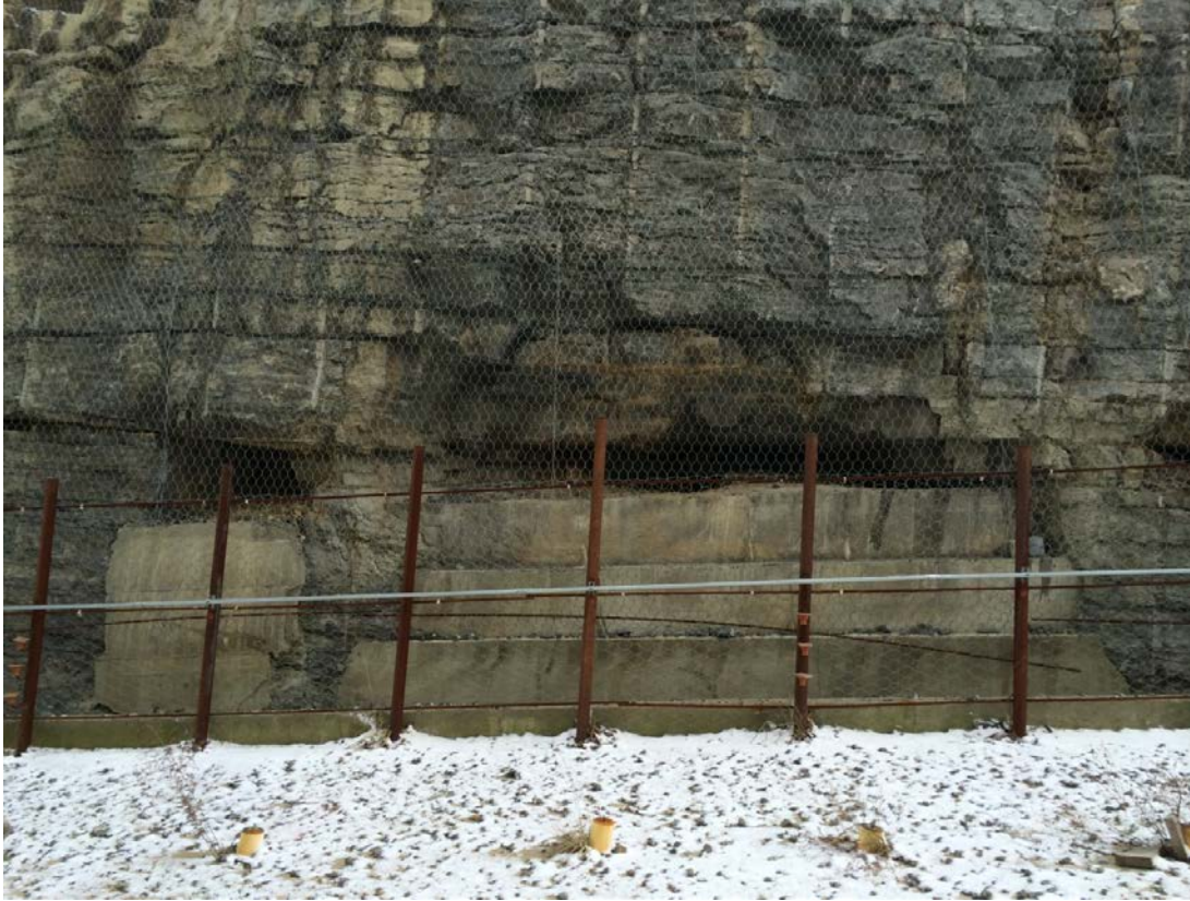
Figure 3-9. View of Karst Feature at Base of Presplit with Concrete Added at Cave Mouth.
