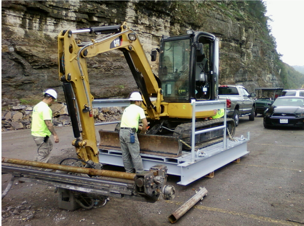
Figure 6-19. View of Drill Attachment with Button Bit Used for Drilling Small Blastholes to Perform Trim Blasting on a Rock Slope.
