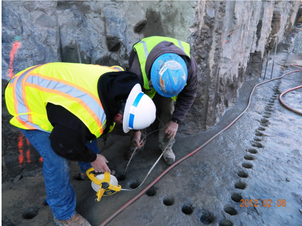
Figure 6-13. Line Drilling Holes on an inside and outside Corner. Crew Checking the Depths to Quality Control (QC) the Drillers Work.
