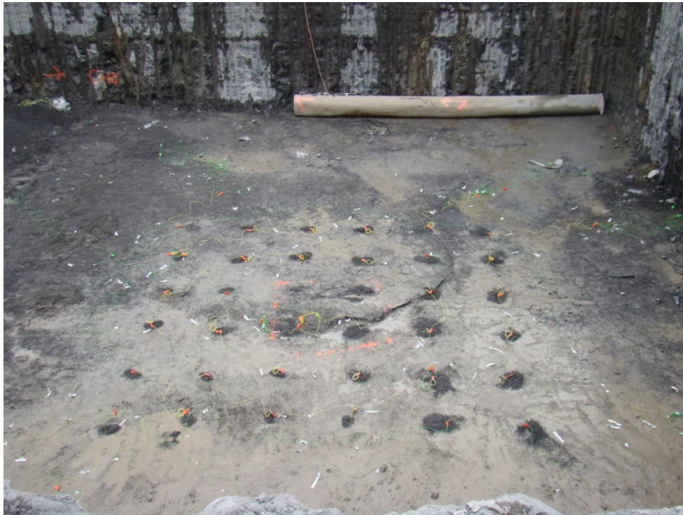
Figure 1-6 Sinking Shot Loaded and Hooked up for Excavating a Lock Monolith Foundation.
