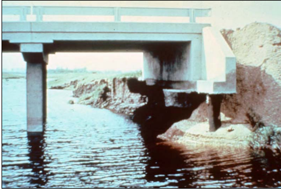
Figure 14.1. Scour of bridge abutment and approach embankment.
