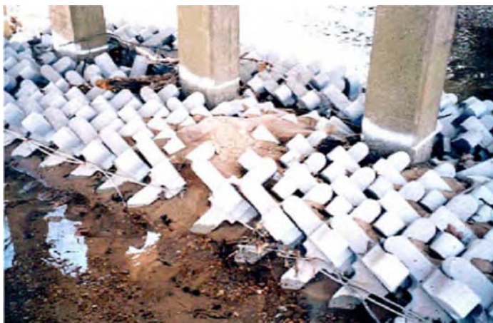
Figure 19.5c. Close-up of armor units after several flow events at Bridge 133, Graves County, KY
