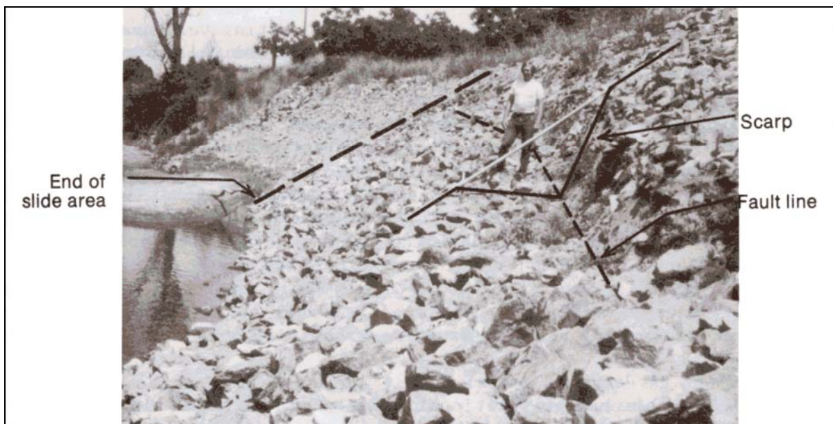
Figure 5.11. Riprap on Cosumnes River at Site 2 near Sloughouse, CA, looking downstream, showing translational slide failure (photographed May 31, 1983) (Blodgett & McConaughy 1986).
