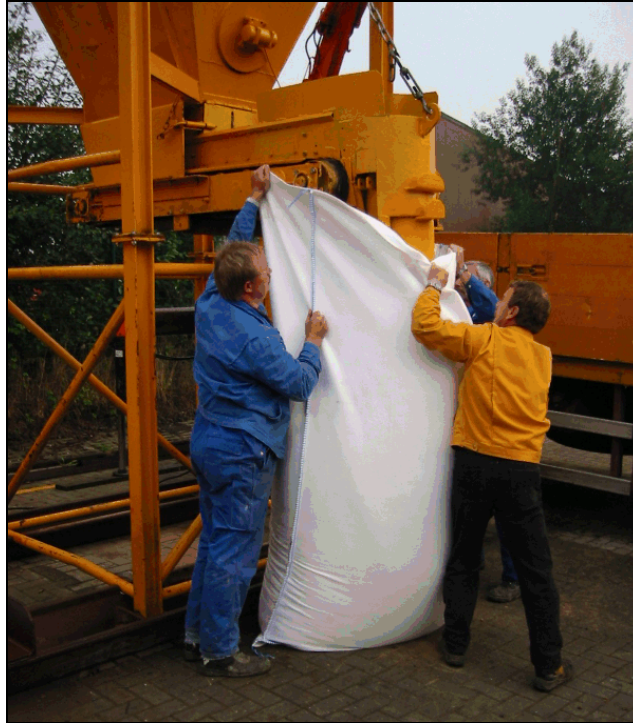
Figure 5.5. Filling 1.0 metric tonne geotextile container with sand. (photo from NCHRP Project 24-07(2), courtesy Colcrete – Von Essen Inc.)
