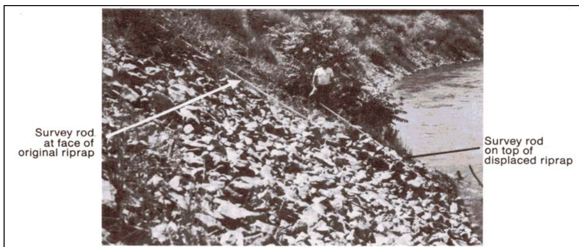
Figure 5.13. Riprap on Consumnes River at Site 3 near Sloughouse, CA, looking downstream, showing modified slump failure (photographed May 31, 1983) (Blodgett & McConaughy 1986).
