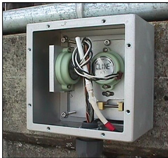
Figure 9.19. Detail of tilt meter.
