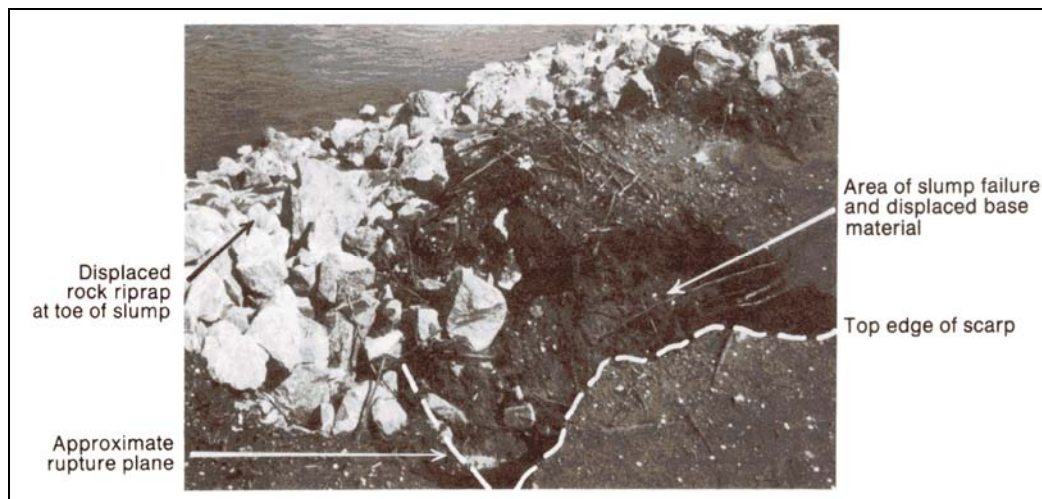
Figure 5.15. Riprap on left bank Cosumnes River at Site 1 near Sloughouse, CA, showing slump failure (photographed May 31, 1983) (Blodgett & McConaughy 1986).
