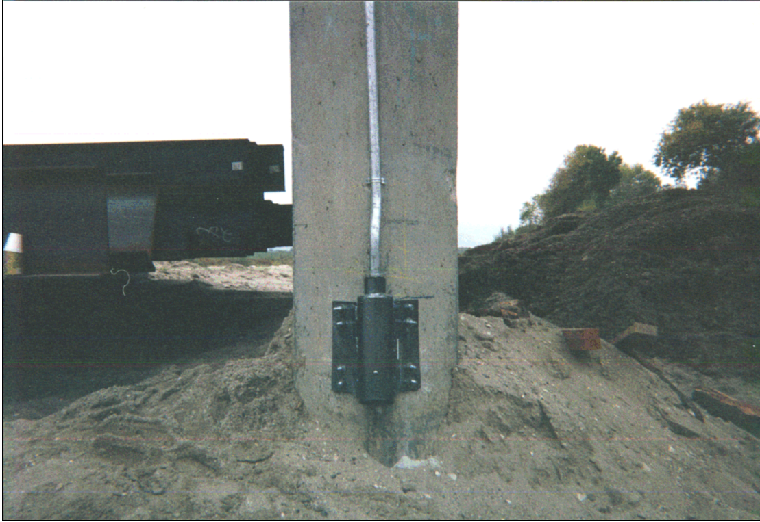
Figure 9.28. Close up of sonar scour monitor on Salinas River Bridge near Soledad, CA.
