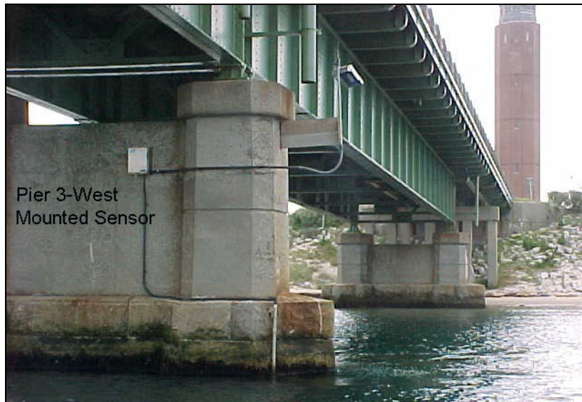
Figure 9.13. Sonar scour monitor installation including remote station and solar panel.
