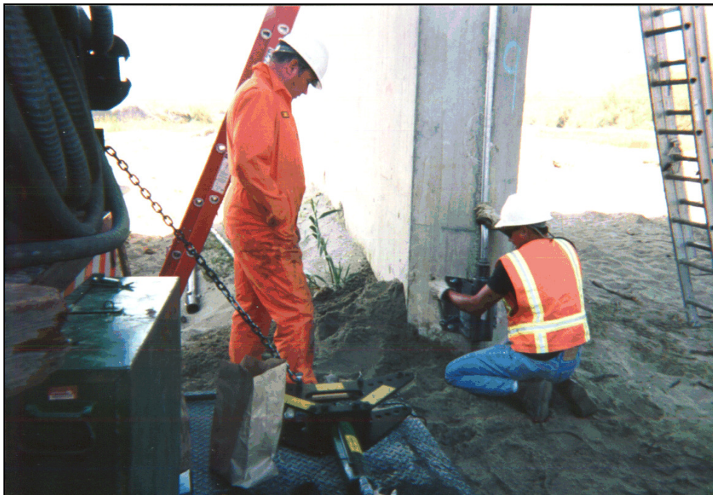
Figure 9.27. Installation of a sonar scour monitor on Salinas River Bridge near Soledad, California (Highway 101) by CALTRANS.
