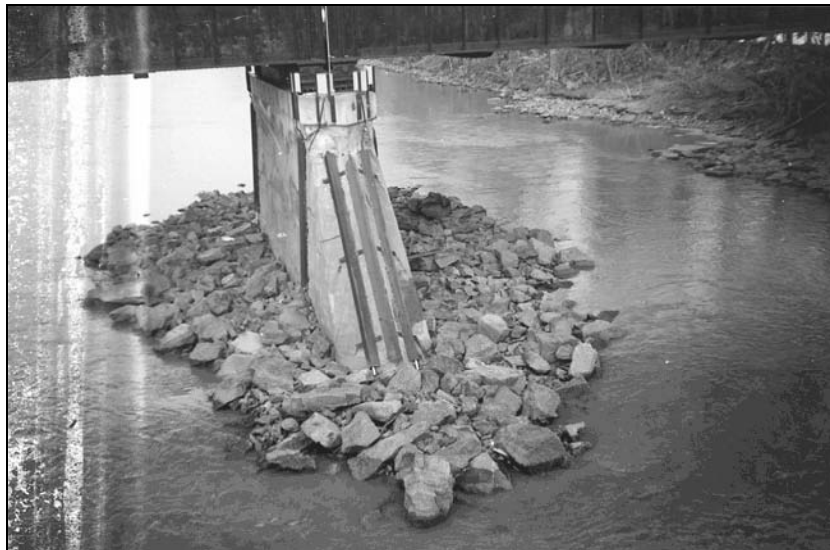
Figure 9.21. Brisco Monitor sounding rods installed at a bridge pier in New York to monitor movement of riprap (Butch 1996).
