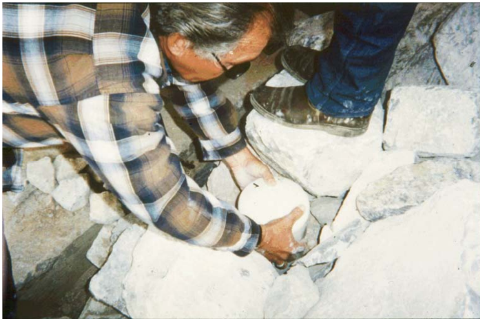
Figure 9.32. Installation of a float out device by Nevada DOT to monitor riprap stability.
