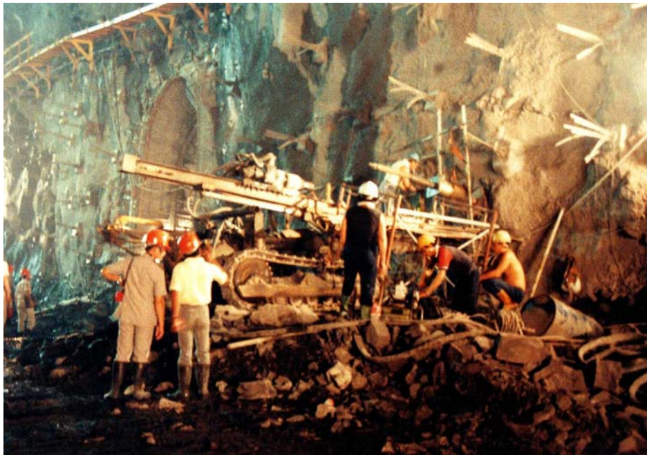
Figure 14.30: Installation of cables in the sidewall of the power cavern in the Mingtan Pumped Storage Project in Taiwan.
