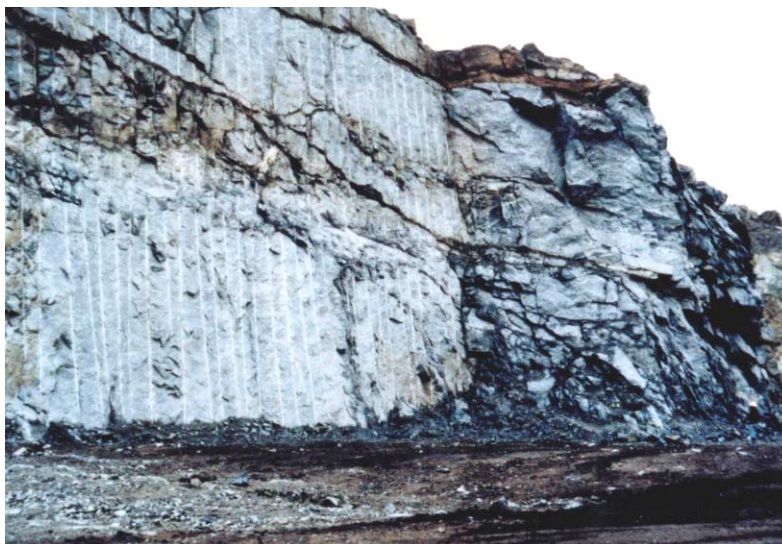
Figure 16.1: Comparison between the results achieved by pre-split blasting (on the left) and normal bulk blasting for a surface excavation in gneiss.
