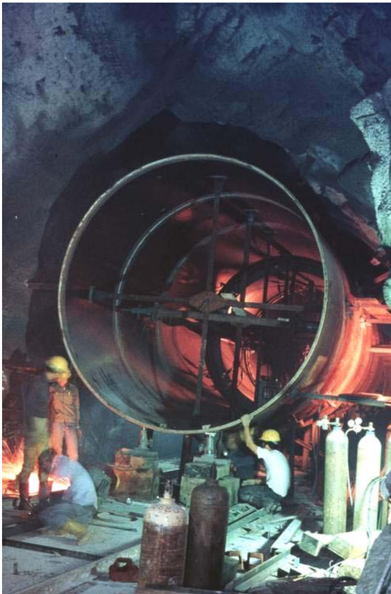
Figure 1.9: Installation of steel lining in a pressure tunnel in a hydroelectric project.
