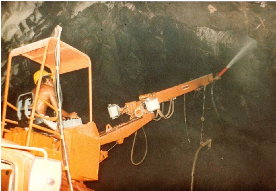
Figure 15.9: A truck mounted shotcrete robot being used in a large civil engineering tunnel. Note that the distance between the nozzle and the rock surface is approximately one metre.
