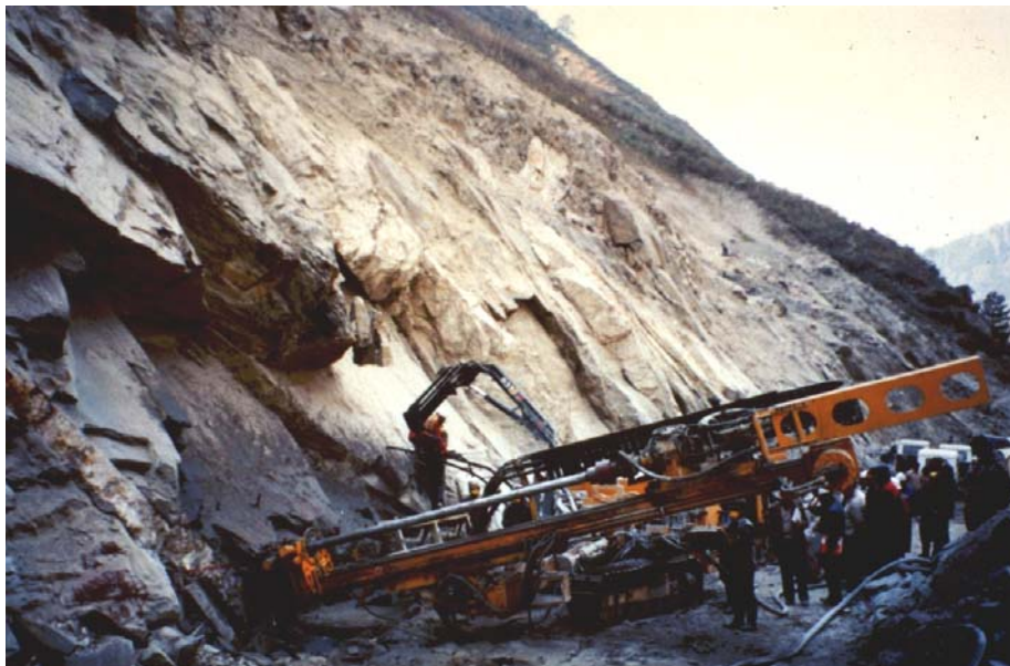
Figure 14.16: Drilling machine for the installation of 40 m long reinforcing cables in 50 mm diameter holes in a dam excavation.
