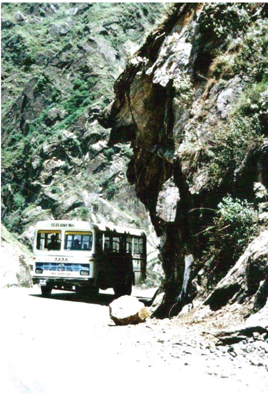
Figure 9.1: A rock slope on a mountain highway. Rockfalls are a major hazard on such highways.
