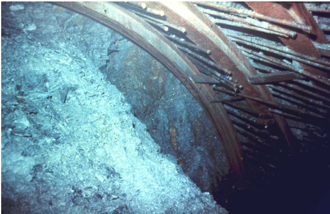
Figure 12.18: Spiling in very poor quality clay-rich fault zone material.
