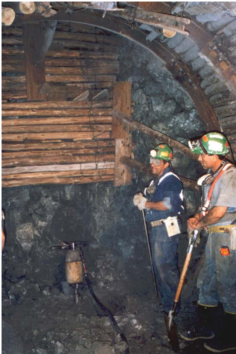
Figure 12.17: Installation of sliding joint top hat section steel sets immediately behind the face of a tunnel being advanced through very poor quality rock.
