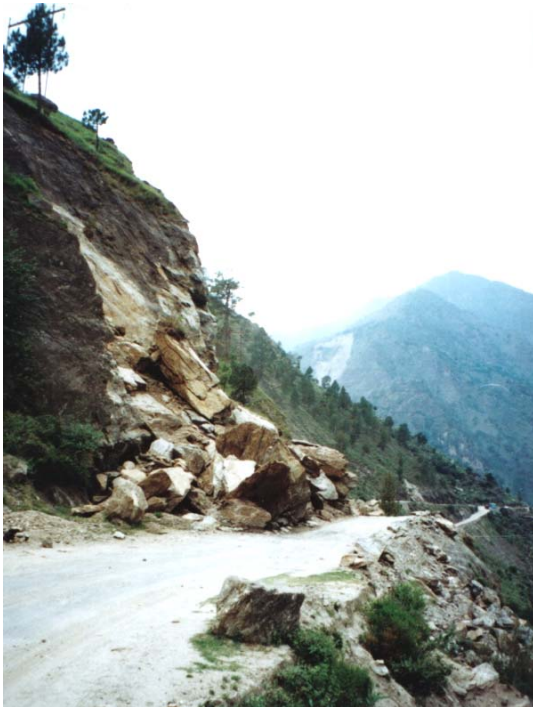
Figure 7.3: A rock slide on a road caused by the undercutting of sheet joints in a granite slope. In hard rocks such as granite, failure can occur very suddenly if the factor of safety of the slope is close to 1. A rise in groundwater levels during a heavy storm or ice jacking in winter may be sufficient to induce failure.
