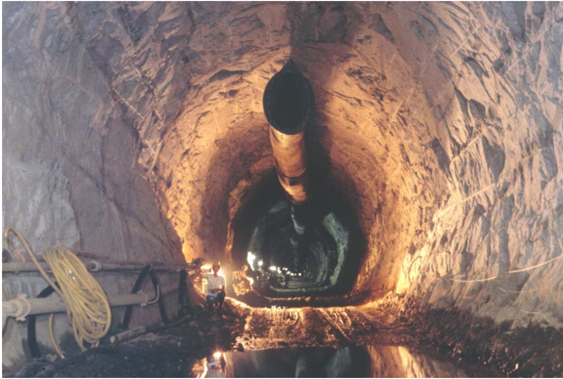
Figure 16.5: Results achieved using well designed and carefully controlled blasting in a 19 foot diameter tunnel in gneiss in the Victoria hydroelectric project in Sri Lanka. Photograph reproduced with permission from the British Overseas Development Administration and from Balfour Beatty - Nuttall.
