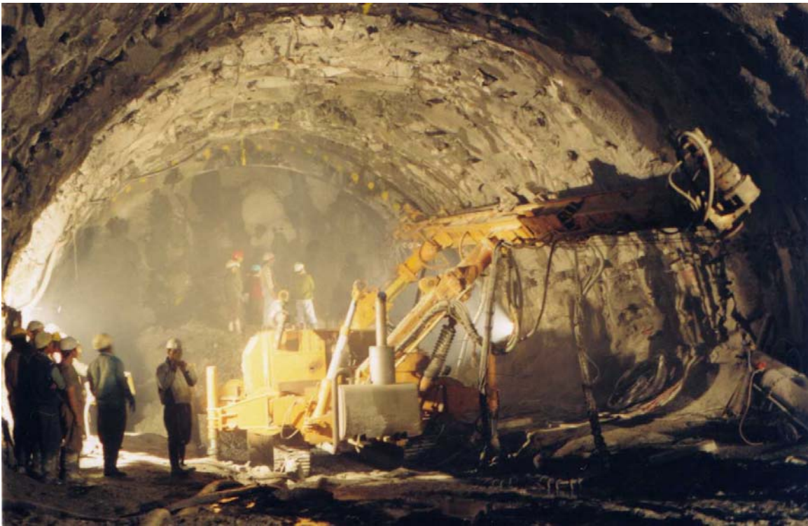
Figure 12.20: Installation of 12 m long 75 mm diameter pipe forepoles in an 11 m span tunnel top heading in a fault zone.
