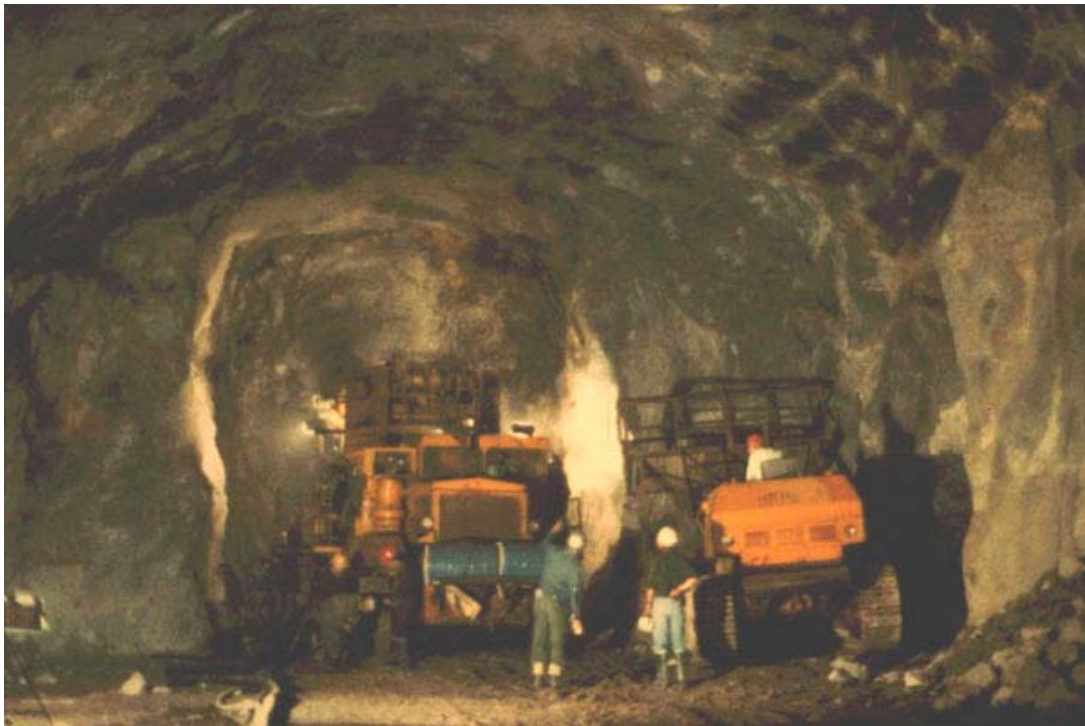
Figure 6.4: A 6 m wide heading driven ahead of the tunnel face to permit pre-reinforcement of potentially unstable wedges in the roof. The seven-boom jumbo is seen working in the heading.
