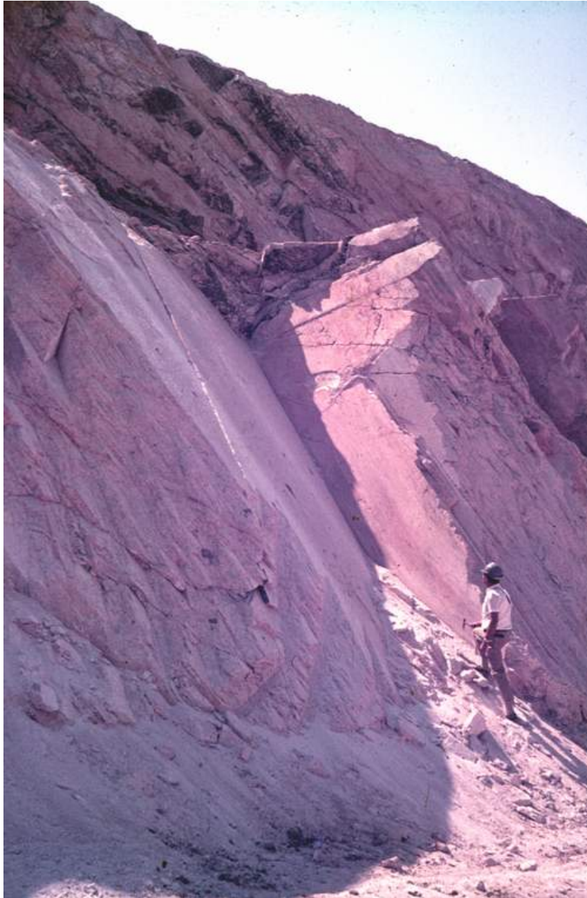
Figure 1.3: A wedge failure controlled by intersecting structural features in the rock mass forming the bench of an open pit mine.
