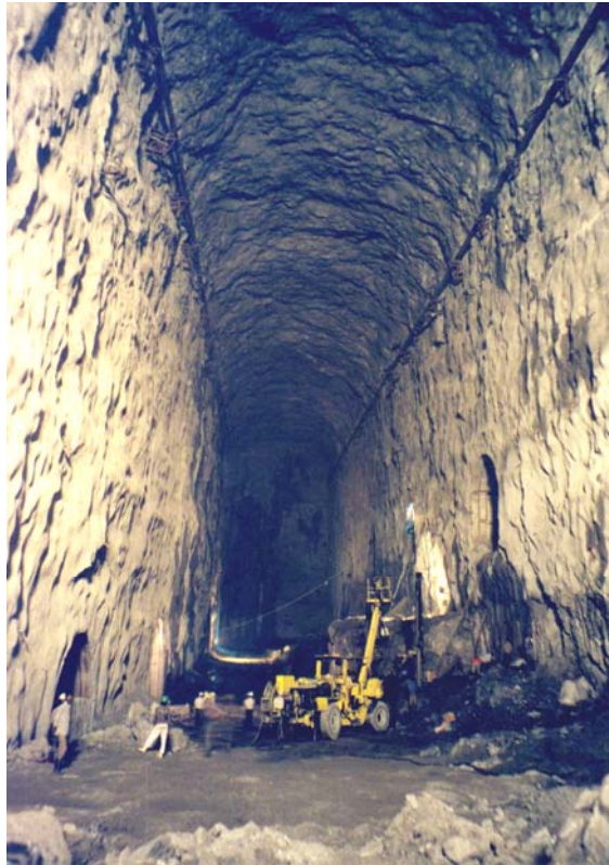
Figure 11.22: Partially completed 20 m span, 42.5 m high underground powerhouse cavern of the Nathpa Jhakri Hydroelectric Project in Himachel Pradesh, India. The cavern is approximately 300 m below the surface.
