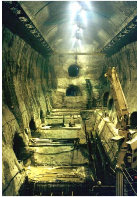
Figure 13.9: Example of suspended crane beams in the powerhouse cavern of the Singkarak Hydroelectric Project in Indonesia.
