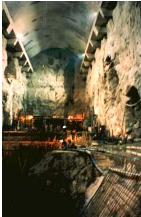
Figure 13.10: Example of anchored crane beams in the underground powerhouse cavern for the Thissavros Hydroelectric project in Greece. In this case the beams shown were used for a construction crane and concrete columns were added later to carry the full crane loads.
