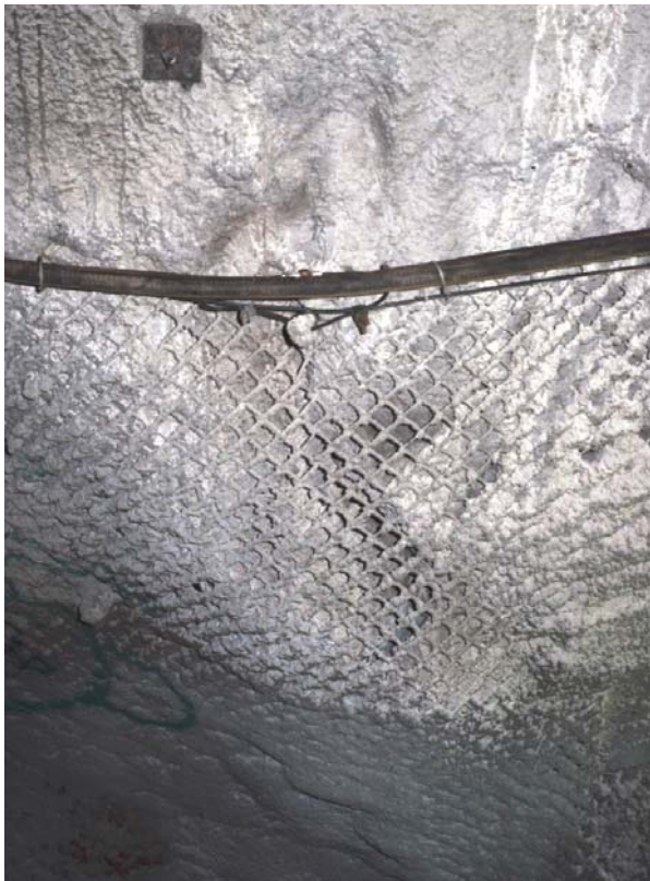
Figure 15.7: Chainlink mesh, while very strong and flexible, is not ideal for shotcrete application because it is difficult for the shotcrete to penetrate the mesh.
