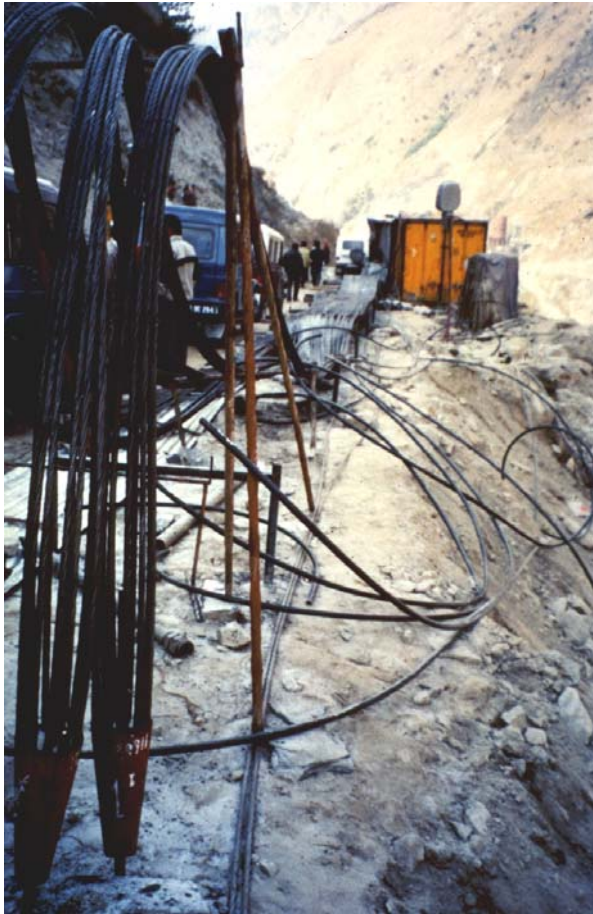
Figure 14.17: 40 m long multi-strand cables with a capacity of 200 tons each being prepared for installation in a dam excavation.
