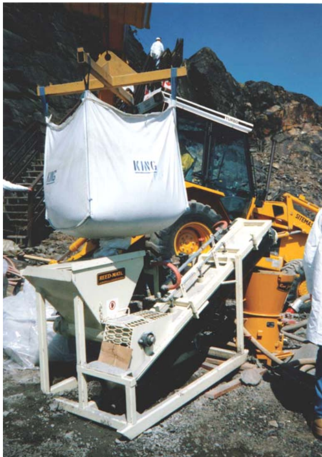
Figure 15.3: Bagged pre-mixed dry shotcrete components being delivered into a hopper feeding a screw conveyor, fitted with a pre-dampener, which discharges into the hopper of a shotcrete machine
