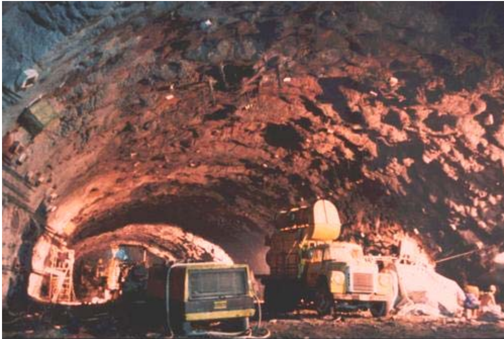
Figure 13.19: Cables and shotcrete were used to support the roof of the power cavern in the Mingtan Pumped Storage Project in Taiwan.
