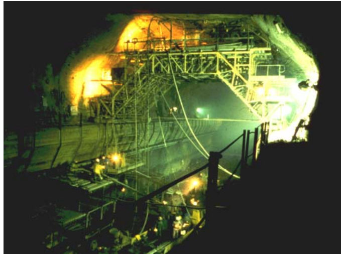
Figure 13.8: Example of a cast in place crane beam in the Drakensberg Pumped storage project in South Africa. The beam is supported against a vertical face of interbedded sandstone, siltstone and mudstone by means of stressed and grouted cables. A temporary construction crane that was used to access the roof is shown in the photograph.
