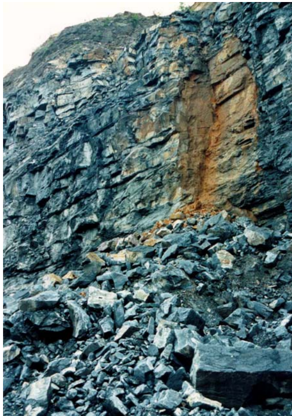
Figure 11.30: Structurally controlled failure in the face of a steep bench in a heavily jointed rock mass.
