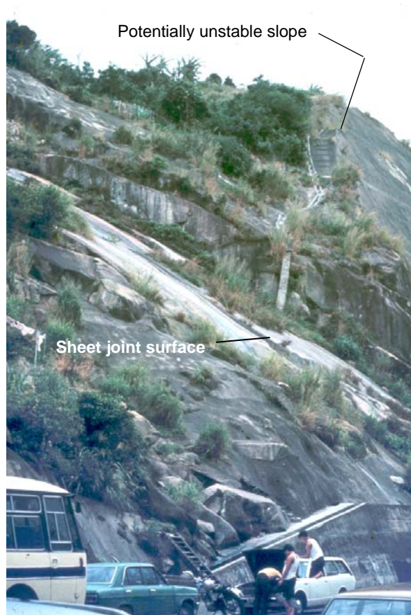
Figure 7.4: The failure surface defined by a sheet joint surface on which a small slide occurred during blasting of the original cut slope for the Sau Mau Ping Road. The potentially unstable slope under consideration is visible in the back-ground.
