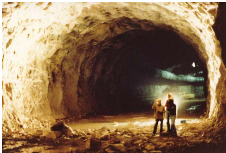
Figure 11.21: Top heading of the 12 m span, 18 m high tailrace tunnel for the Rio Grande Pumped Storage Project.
