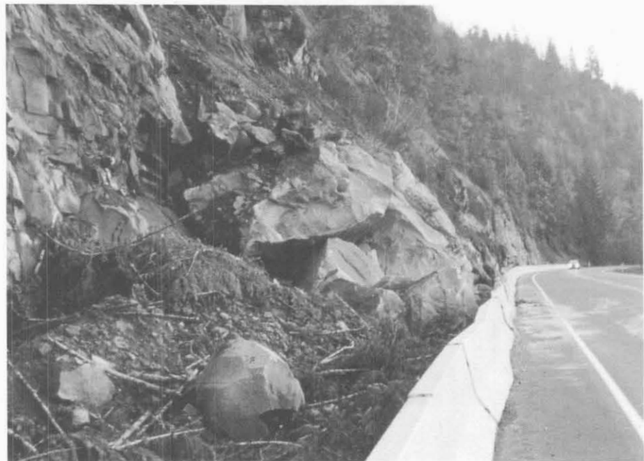
Figure 8.2: When the large block fell, some of the debris reached the roadway. Future rockfalls, which will be smaller, should be retained in the ditch.
