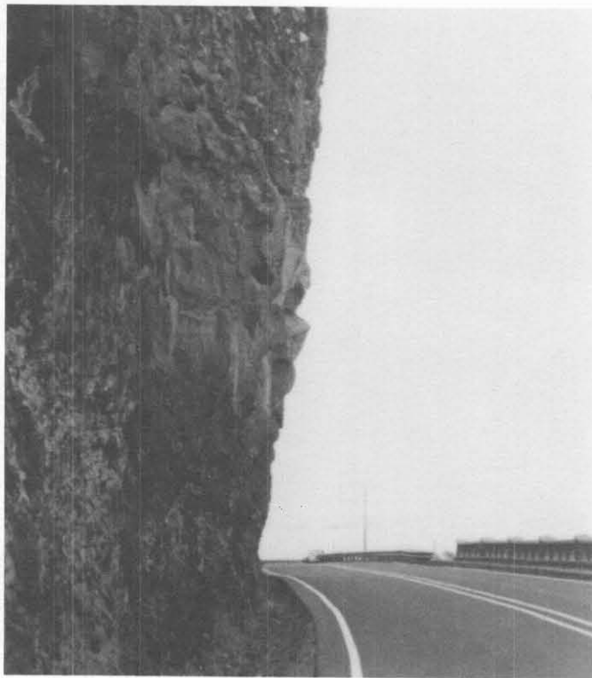
Figure 5.6 Rockfall from this slope will land on the roadway. No catchment is provided by the ditch.
