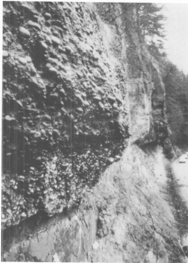
Figure 3.6 Ineffective roadside ditch.
