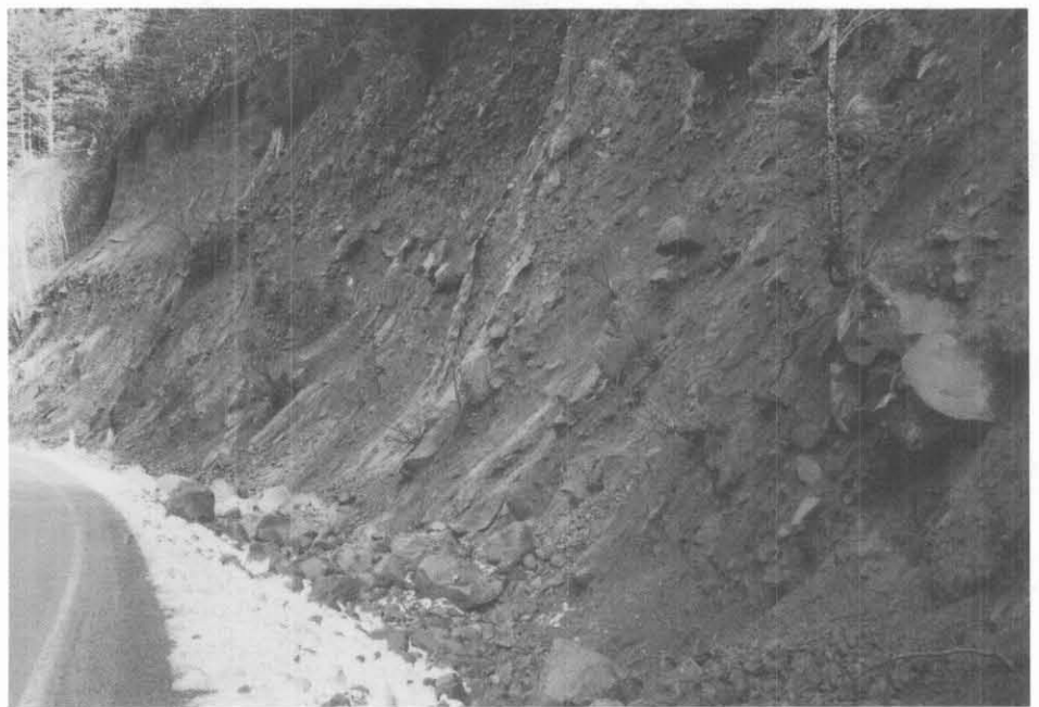
Figure 5.25 Oversteepened soil/rock slope
