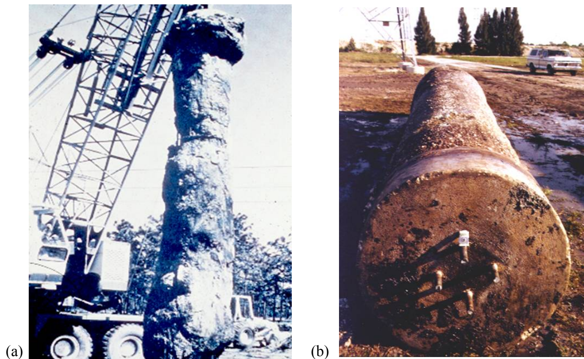
Figure 9-57. Photographs of exhumed shafts (a) shaft where excavation was not adequately cleaned, (b) shaft where excavation was properly cleaned (FHWA, 2002d).
