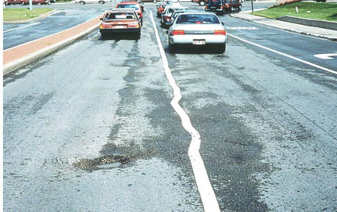
d) Drainage problems
