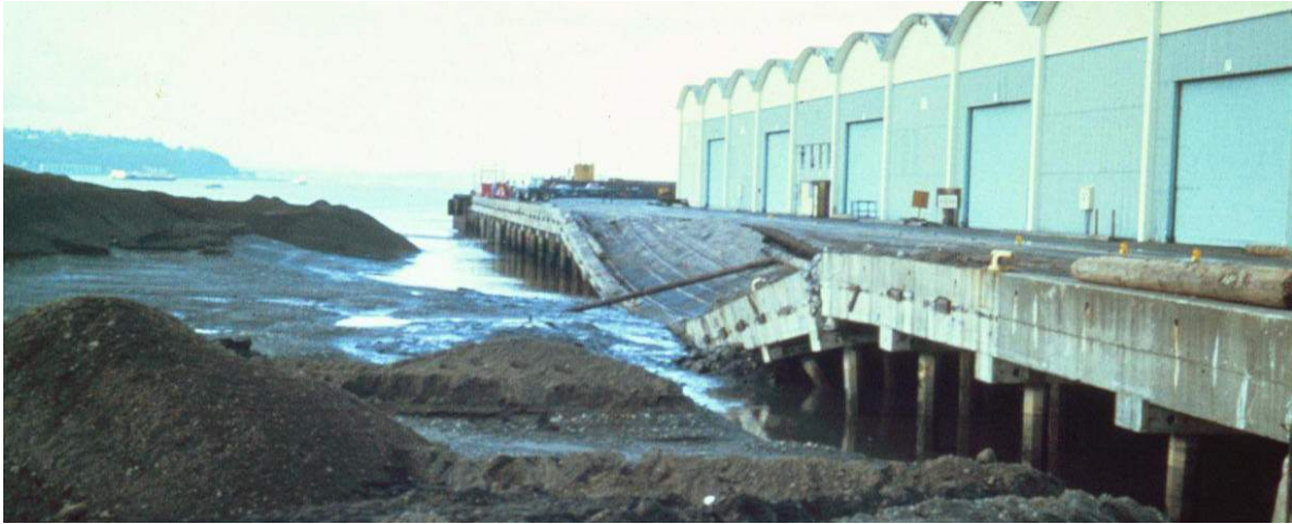
Fig. 7.35 View of the consequence of a hydraulic fill of fine silt flowing against 24-inch piles
