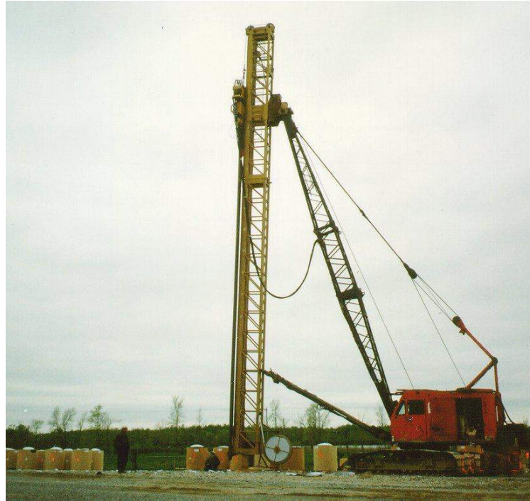
Fig. 4.9 Installation of wick drains type Alidrain (courtesy of J.C. Brodeur, Burcan Industries Ltd.)
