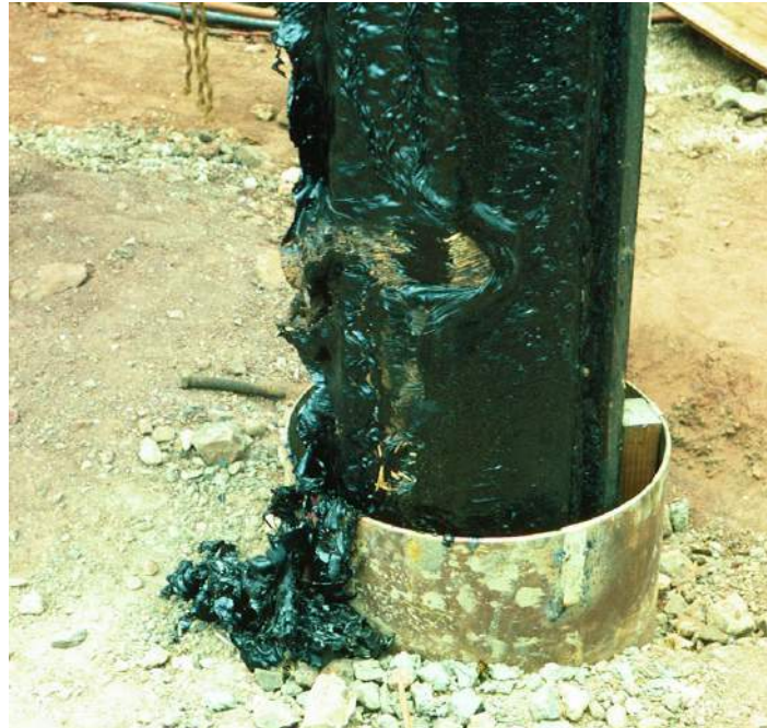
Fig. 7.34 View of a bitumen-coated pile driven through a protective casing The left side of the pile was the pile underside in storage
