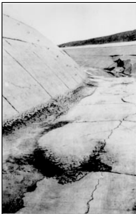
Figure 1-30.—Heaving of canal bottom (about 300 mm at center), Mohawk Canal, Arizona.
