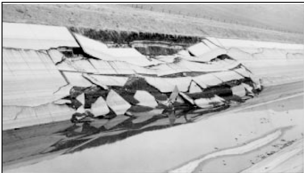
Figure 1-29.—Slope failure and bottom heaving of Friant-Kern Canal, California.
