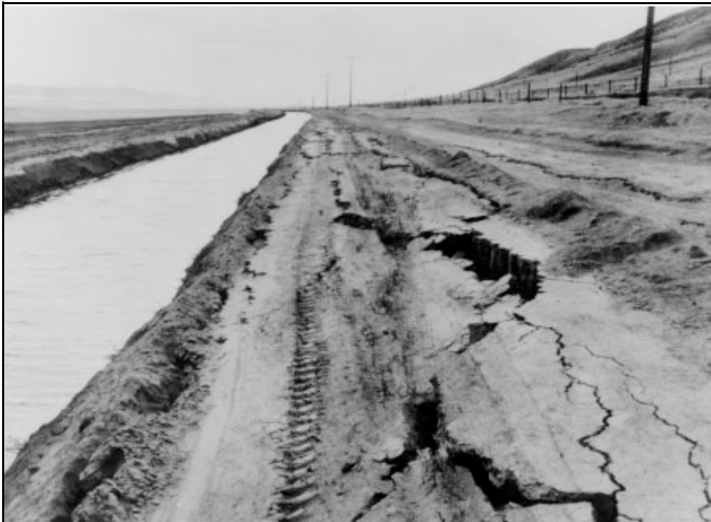
Figure 3-8.—Cracking and settling of canal bank in dry, low-density silt.
